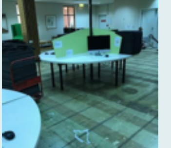
Law Library ceiling after rain
